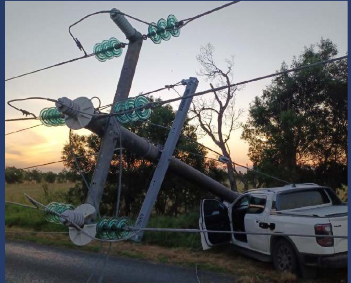
Fallen powerline due to a car collision still live 1 metre off the ground
